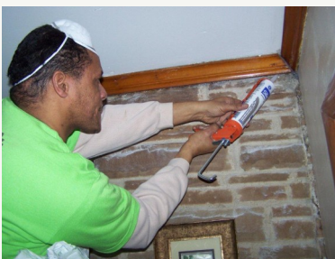
MISSION GREEN TRAINEE IMPROVING THE ENERGY EFFICIENCY OF A HOME ON FORT CAMPBELL.
